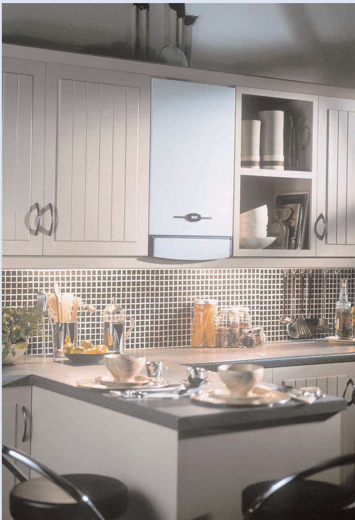
Photograph of wall-hung boiler located in kitchen (courtesy of Baxi Potterton)
