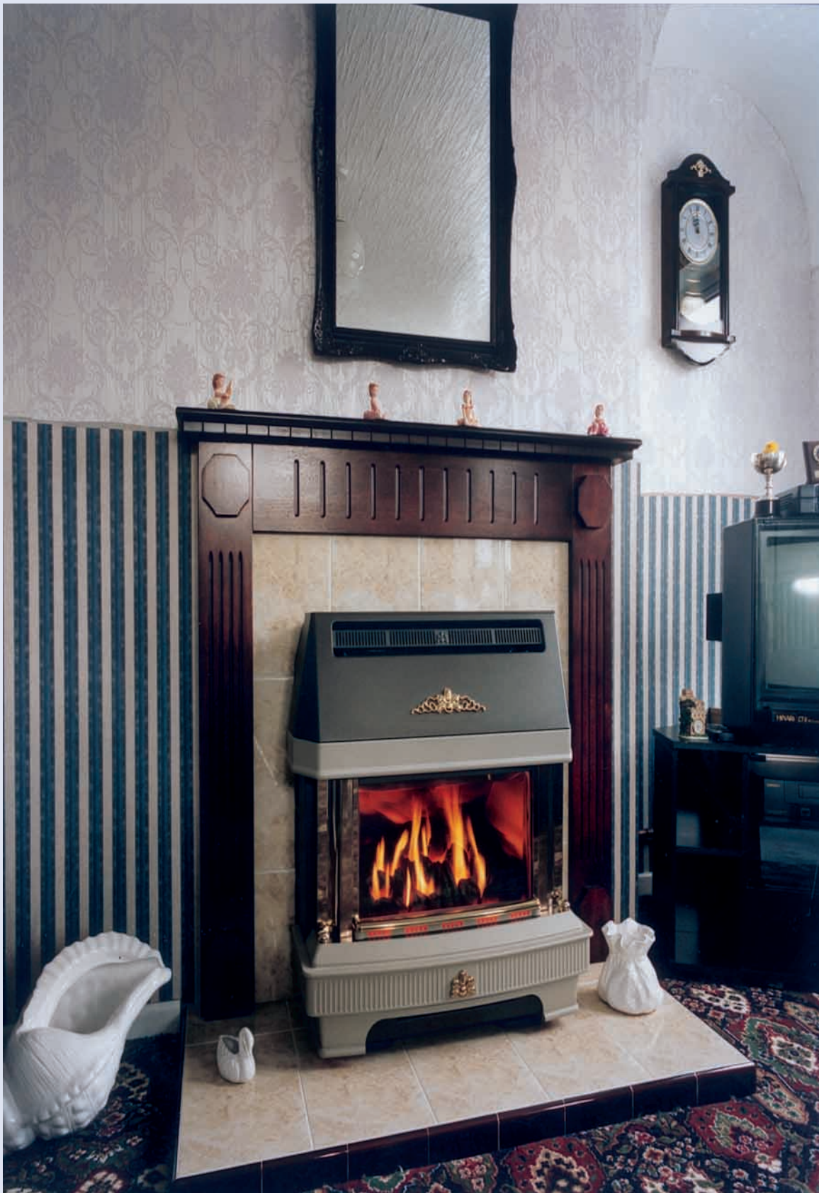
Housing Executive property showing back boiler with fire inset (photo courtesy of NIHE)
